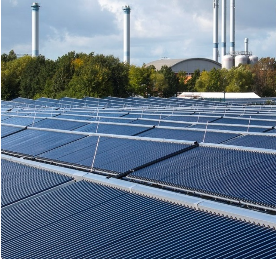
iKWK-System Greifswald (18.732 m 2 ) (Foto: Guido Bröer)
